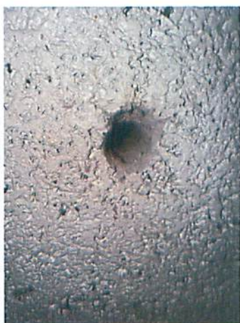
Photograph of core assessment in hempcrete blocks. Block composition turns to clay when drilling. August 13, 2026
