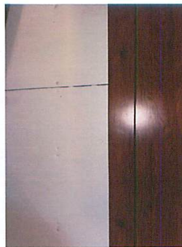
Photograph showing sections of unfinished drywall in basement behind wood panelling. August 13, 2026
