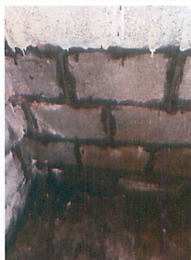
Photograph of unpainted section exposing true composition of foundation to be hempcrete blocks. Blocks were core assessed and found to be solid. August 13, 2026
