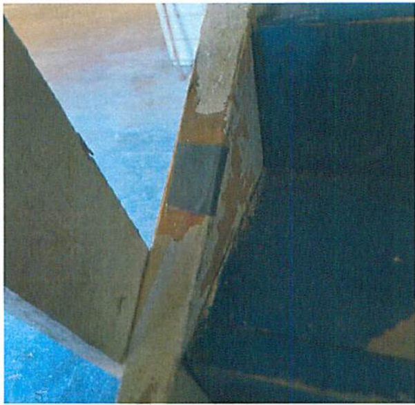
White Paint on rails of stairs
