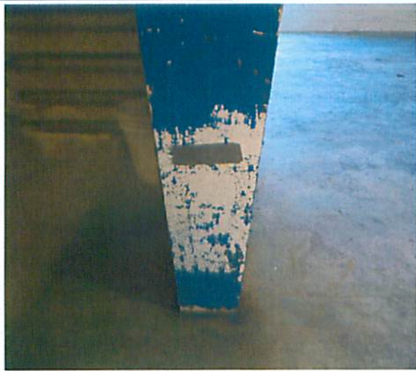
Blue Paint on wall and stairs
