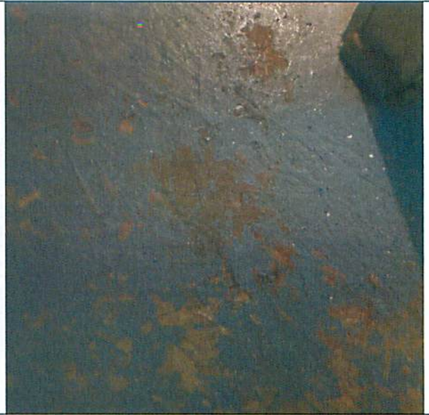
Grey Paint on floor o Mezzanine
