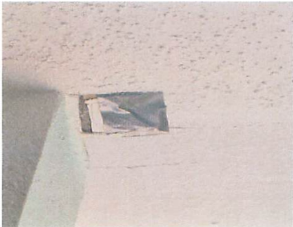
Ceiling Texture in Basement
